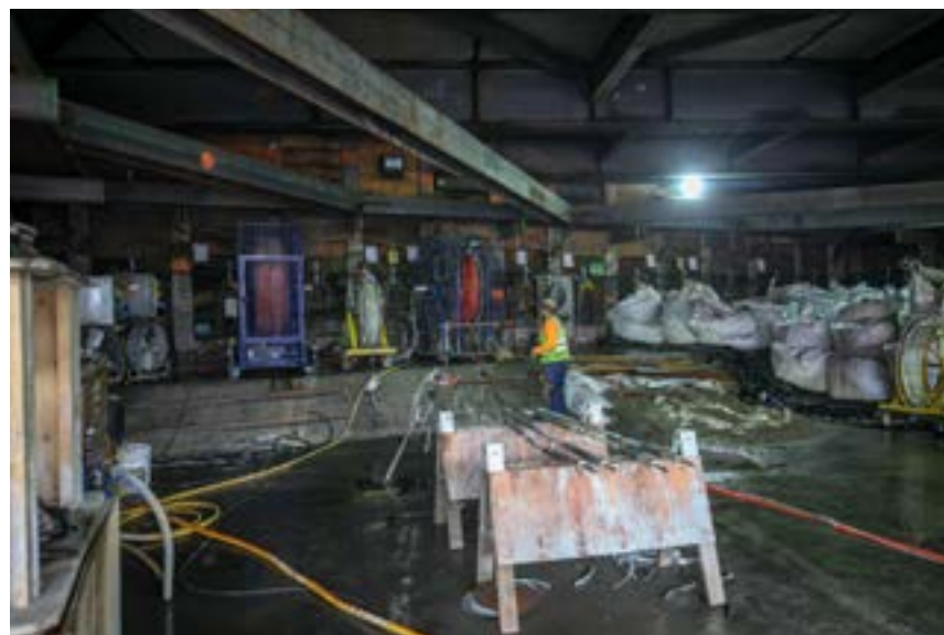
Grout injection through horizontal directionally drilled compensation grout pipes that follow the curvature of the tunnel.
