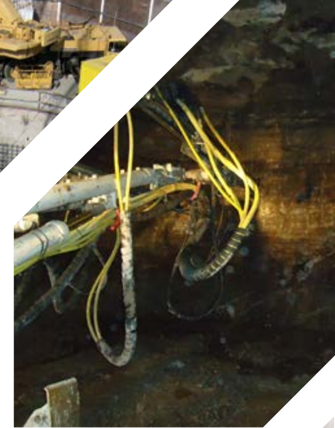
A suite of grout mixes was used to grout highly variable karst rock to perform drill and blast tunneling without water inflow.
